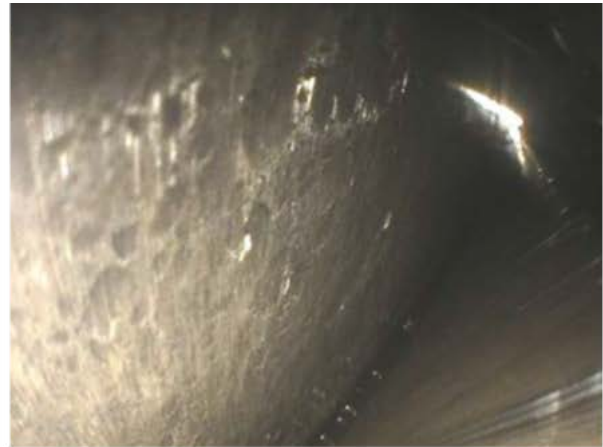
Picture 2 Bad condition of HSS RS bearing outer race and rolling elements.
